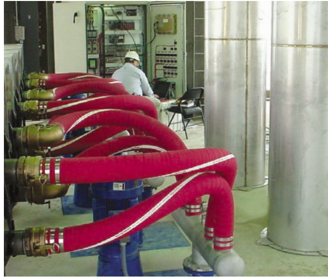
The Gilbert and Mosley groundwater treatment system includes over 5 miles of HDPE piping and a hydraulic-venturi air stripper.
