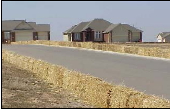
This construction site incorporates Best Management Practices (BMPs). The barriers allow water to drain but prevent silt from flowing into the storm drainage system and ultimately into the streams and rivers.
