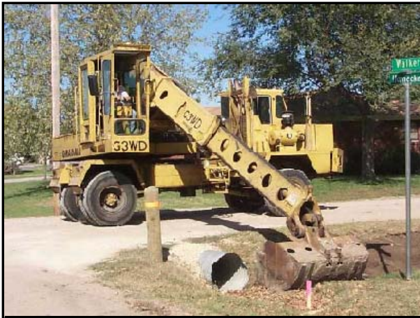
This gradall is one of more than 250 pieces of heavy equipment maintained by Fleet.
