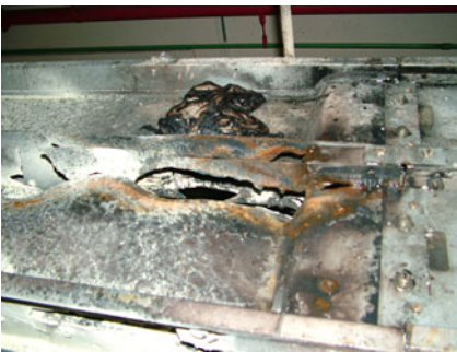
Close up of electrical buss that exploded.
