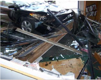
Damage at Rockwell Library
