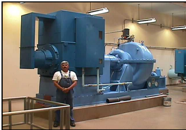
Water is delivered to citizens, thanks to dedicated staff and investments in equipment such as this 2,000 horsepower pump at Hess Pump Station. This pump alone handles approximately 30,000 gallons of water per minute.
